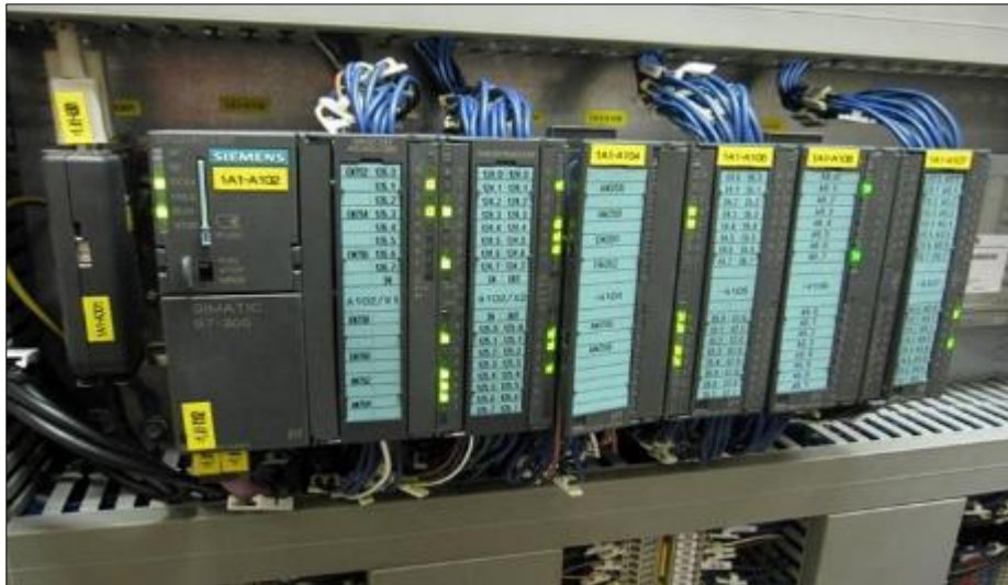
Figure 1 A Programmable Logic Controllers (PLC) [1]
