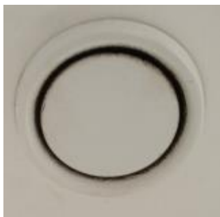
Figure 11 Aspergillus niger on a part of the ventilation system in the locker room at H. Kikić Primary School
