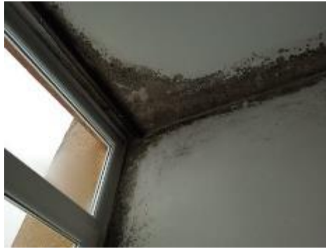
Figure 3 Stachybotris chartarum on the ceiling and wall in A. Šantić Primary School.
