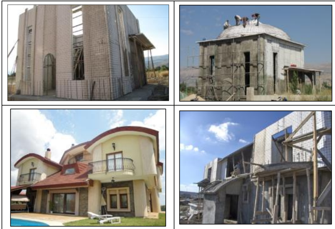
Figure 1 Use of 3D panel in construction of one or two storey buildings
